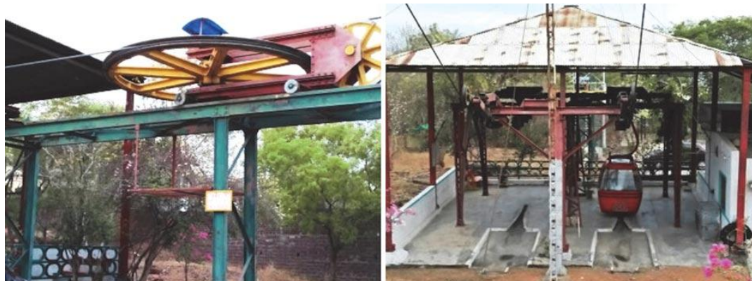
Figure 6- Mechanical System and Passenger Cabin of Bhopal Ropeway at Manuabhan Tekri (photo by authors)
